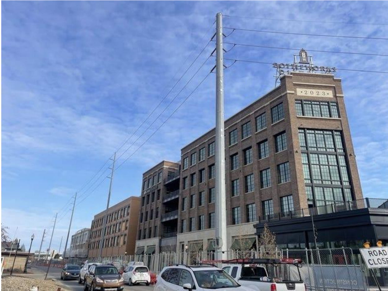
Phase II of the Bottleworks district is seen under construction on Dec. 12, 2024. Alysa Guffey / IndyStar
